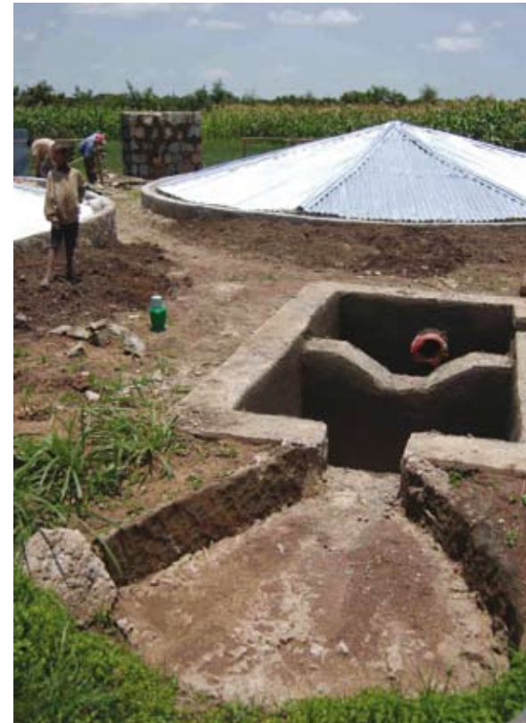
A water-harvesting and underground water storage cistern under construction. Once linked to a micro-irrigation system, farmers will be able to diversify and intensify their production.
